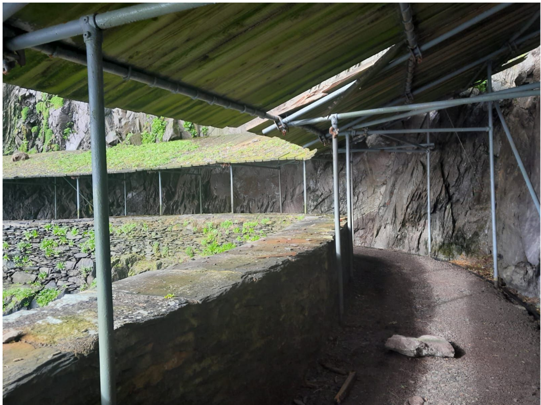
Figure 33 - View of the rock fall at Cross Cove and the damage to the timber decking
