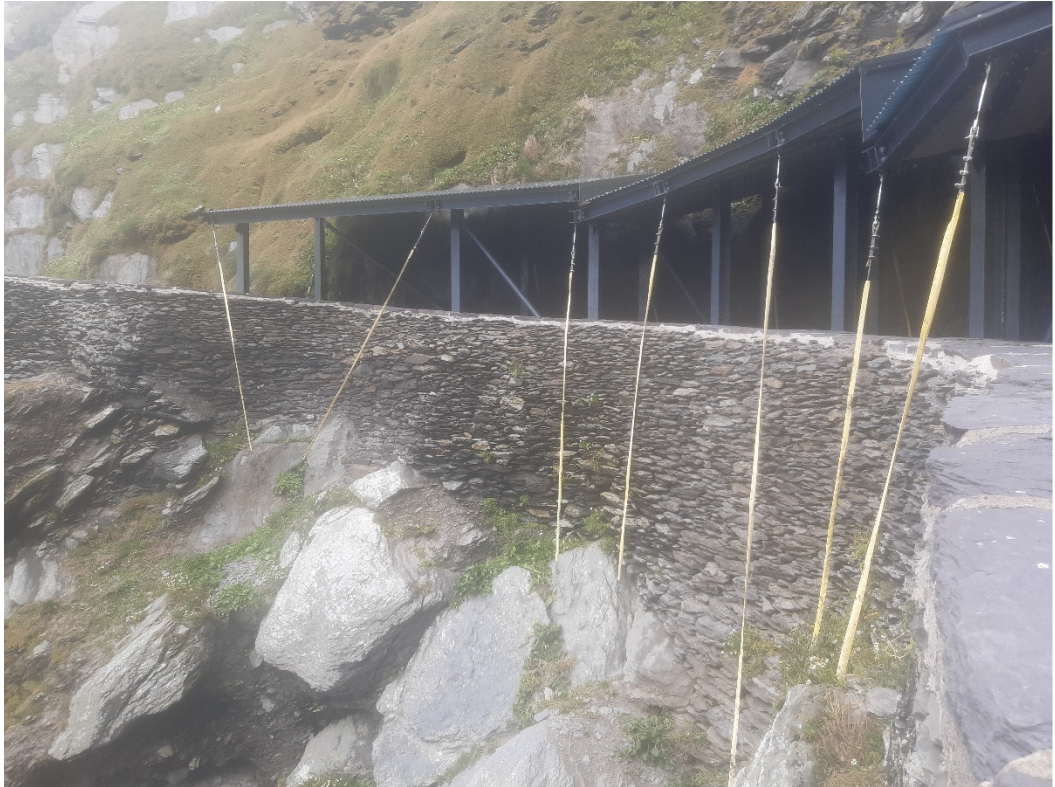
Figure 31 - View of the re-instated stainless steel stays of Crash Deck no. 2 at the end of the season
