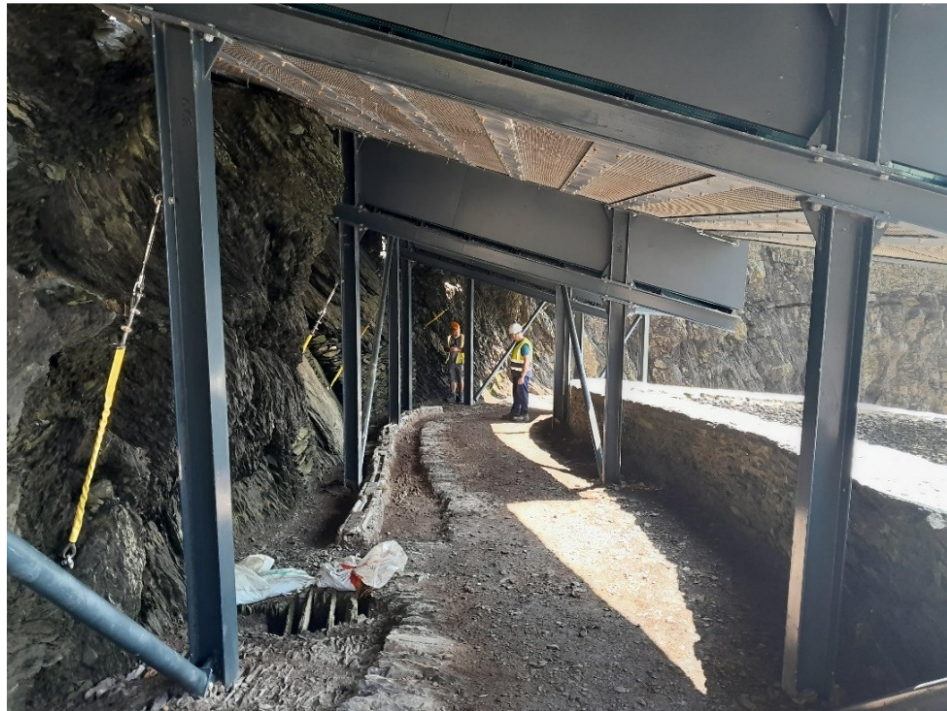
Figure 9 - View of the re-instated historic drains in the location of Crash Deck no .3
