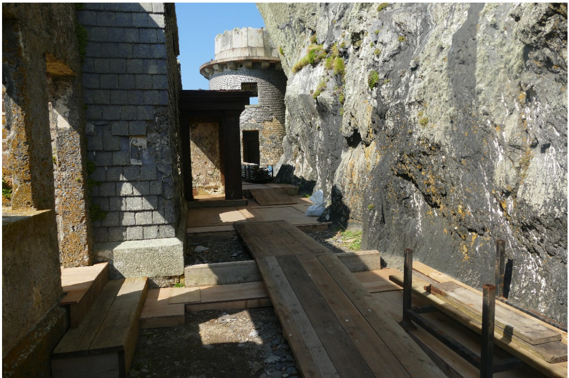
Figure 16 - View of the new installed plywood protection to the existing floor at the upper lighthouse
