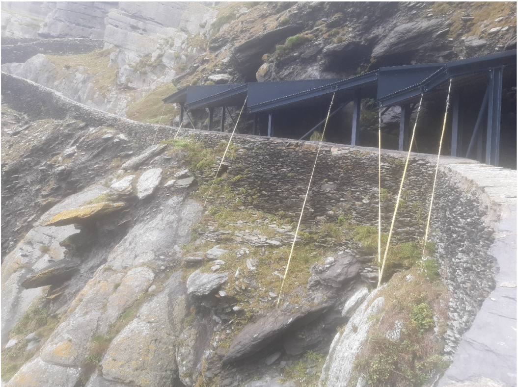
Figure 32 - View of the re-instated stainless steel stays of Crash Deck no. 3 at the end of the season
