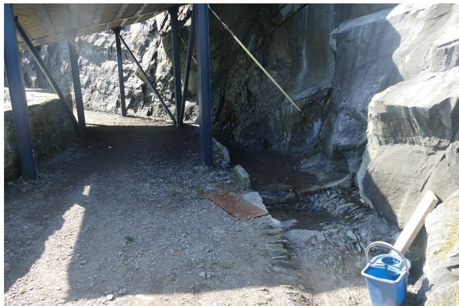
Figure 10 - View of the re-instated historic drains in the location of Crash Deck no .3
