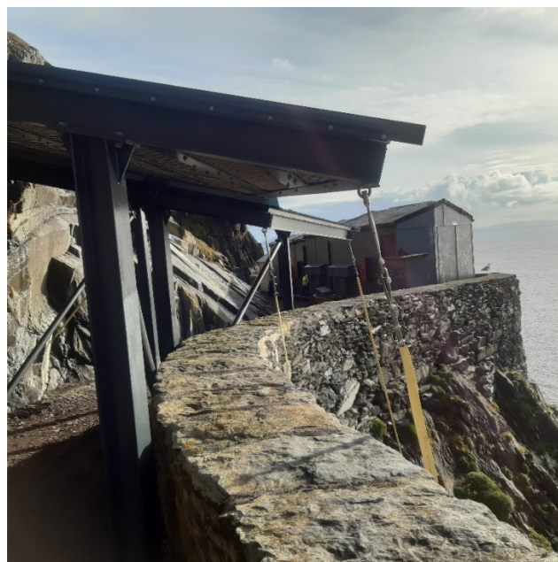
Figure 30 - View of the re-instated stainless steel stays of Crash Deck no. 1 at the end of the season
