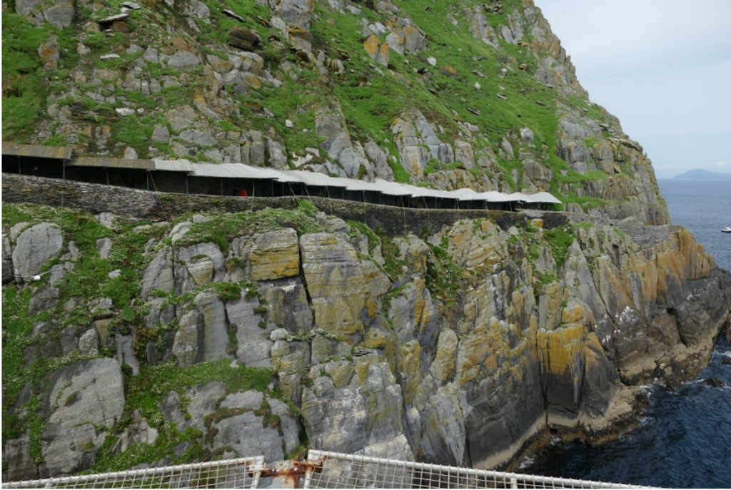
Figure 28 - View of the canopy installed at the Lower Lighthouse road following the rock fall that occurred on 13 th June 2022
