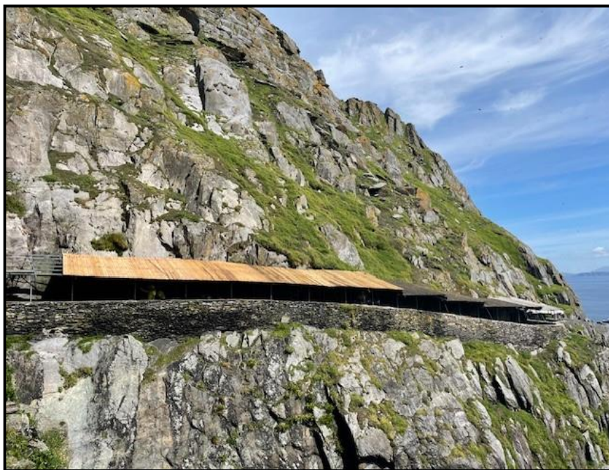
Figure 4 Crash deck at Cross Cove with replacement timbers on roof.
