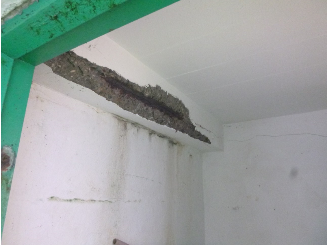
Photo 5: Cracking and exposed rebar in downstand beam of room off entrance
