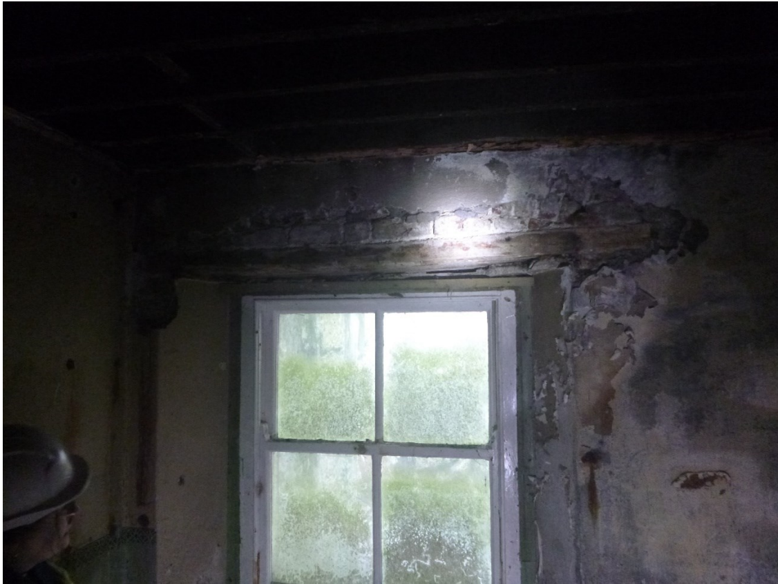
Photo 7: Sagging timber lintel over ground floor window
