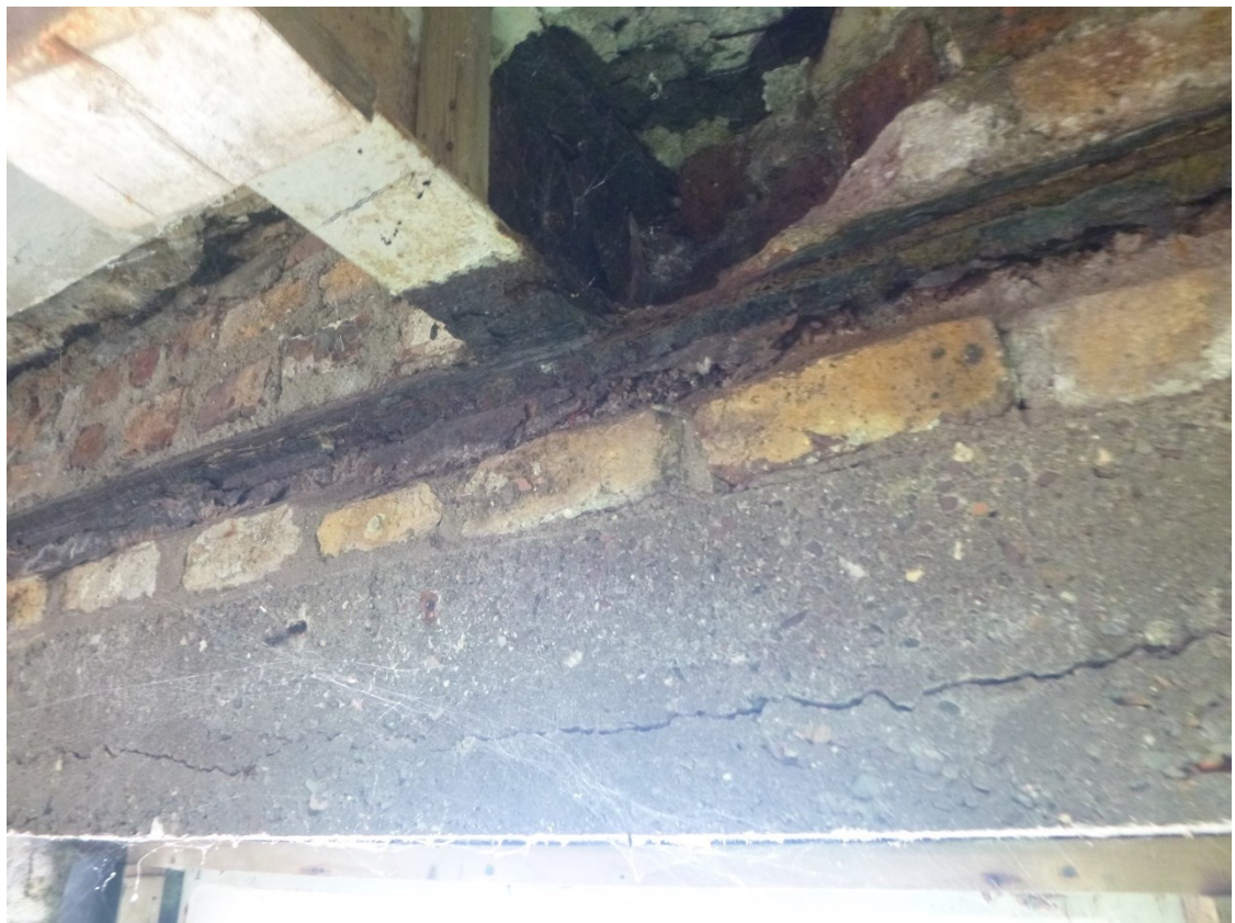
Photo 18: RSJ supporting roof slab bearing onto corroded steel spreader in front wall
