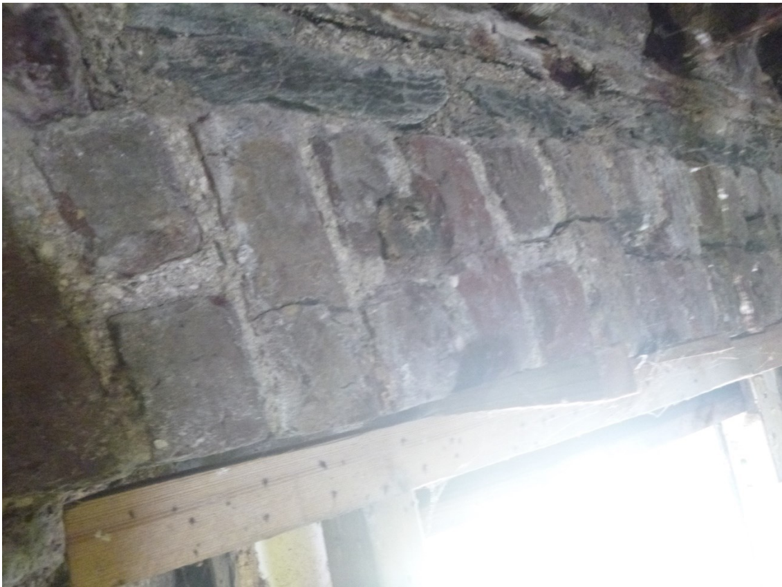
Photo 8: Cracking of bricks in ground floor window lintel
