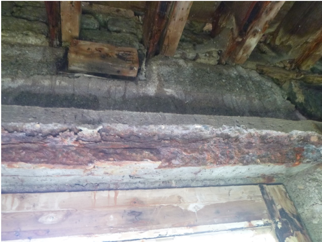
Photo 6: Cracking and corrosion of rebar in ground floor window lintel
