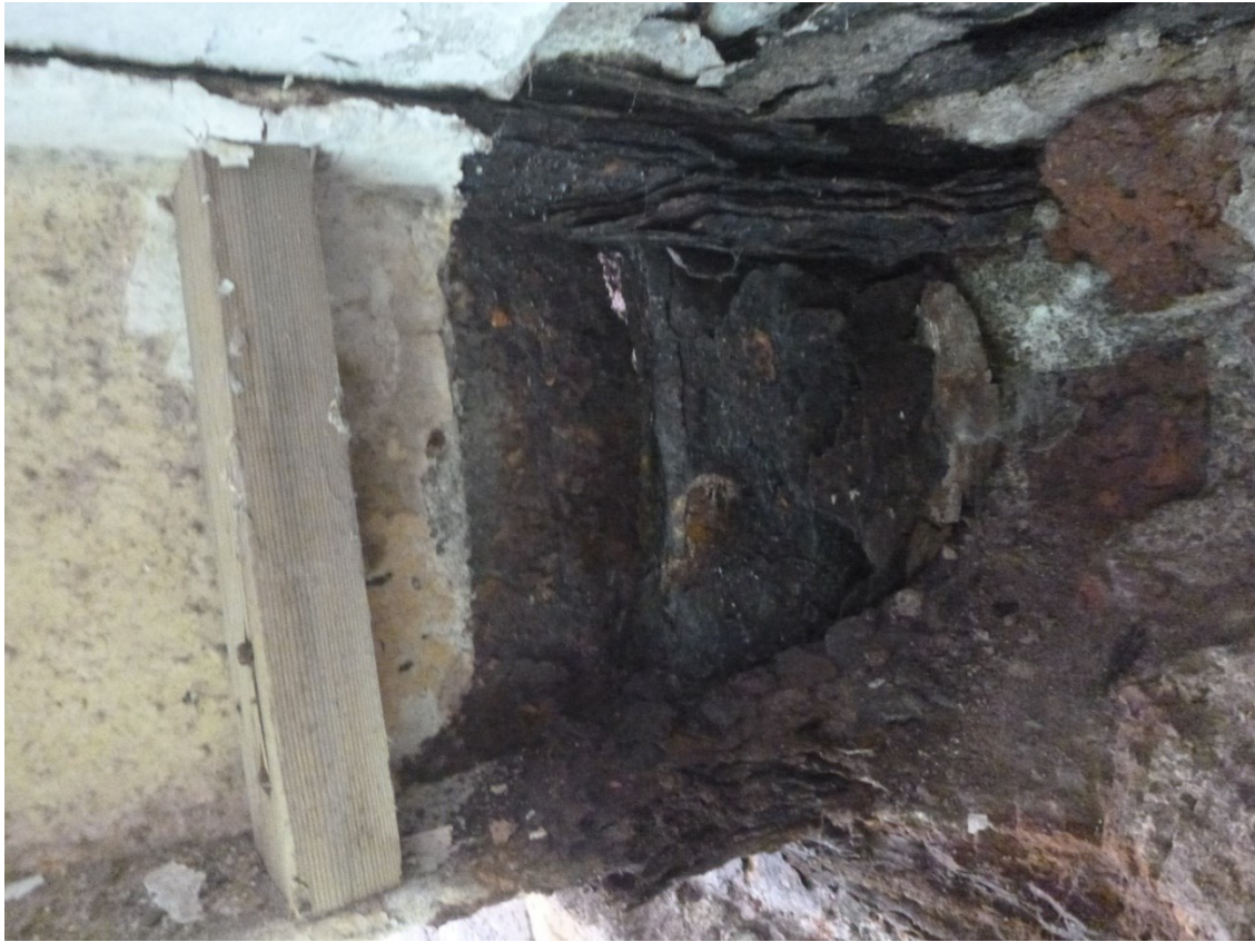
Photo 21: Corrosion of end of roof RSJ built into front wall
