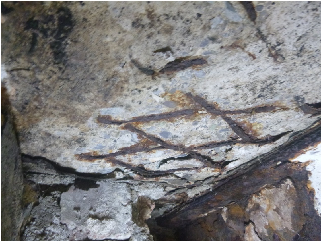
Photo 16: Close up view of corrosion of expanded metal in first floor roof slab
