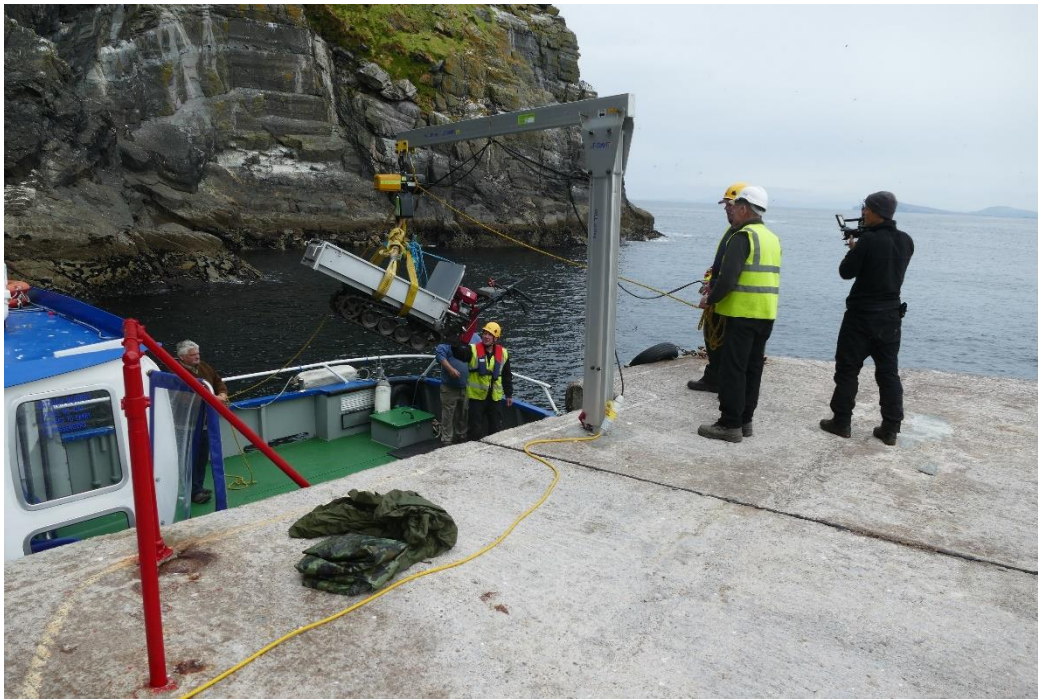
Figure 33 - View of the demountable hoist at the landing pier
