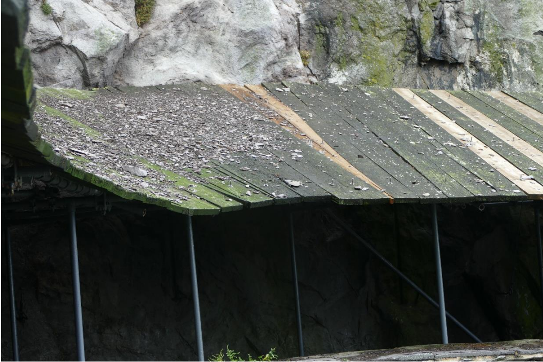
Figure 11 - View of fallen debris on the decking of the protective canopy on the Lower Lighthouse Road
