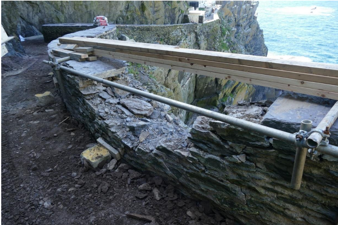
Figure 13 – Example of temporary safety railing installed at the Upper Lighthouse Road by OPW in the 2022 season
