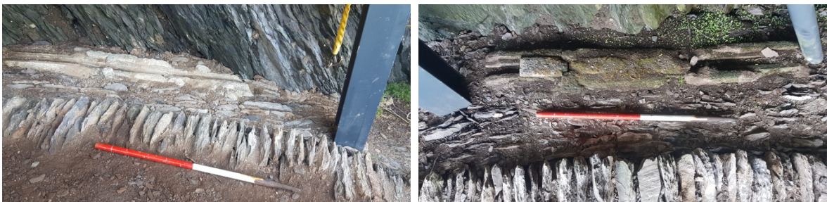
Figs. 11 & 12. Crash Deck 2, details of reinstated cable channel sections sunken into reinstated lateral drain.
