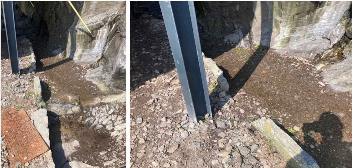
Figs. 7 & 8. Crash Deck 1, the remaining gap in the wall of the 'duckpond'.
