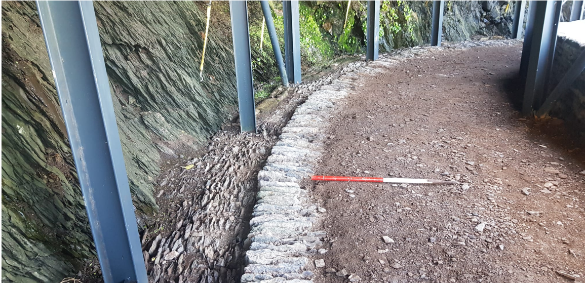
Fig. 9. Crash Deck 2, reinstated road edging, cable channel and lateral drain, looking downhill.
